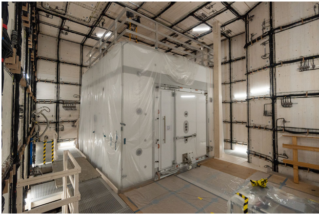
Fig. 15 Photograph of the AMS coil system constructed on the walls of the thermohouse around the MSR. On the right-hand side, in the middle tiles, and on the back-side to the left of the MSR, a few DIN rails are visible which are wired to connect circuits, as explained in the main text. Of course, the AMS extends fully around the MSR, also on the entire floor. The platform visible in front of the MSR is about 2.5 m above floor level
