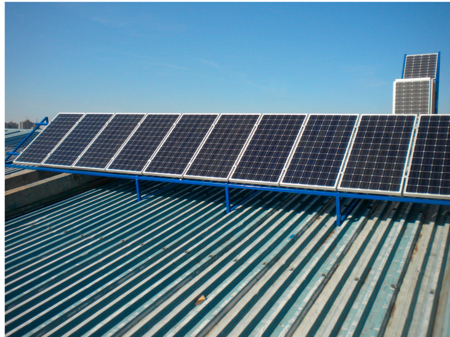
Figure 1. PV array installed on the roof of the faculty [39].
